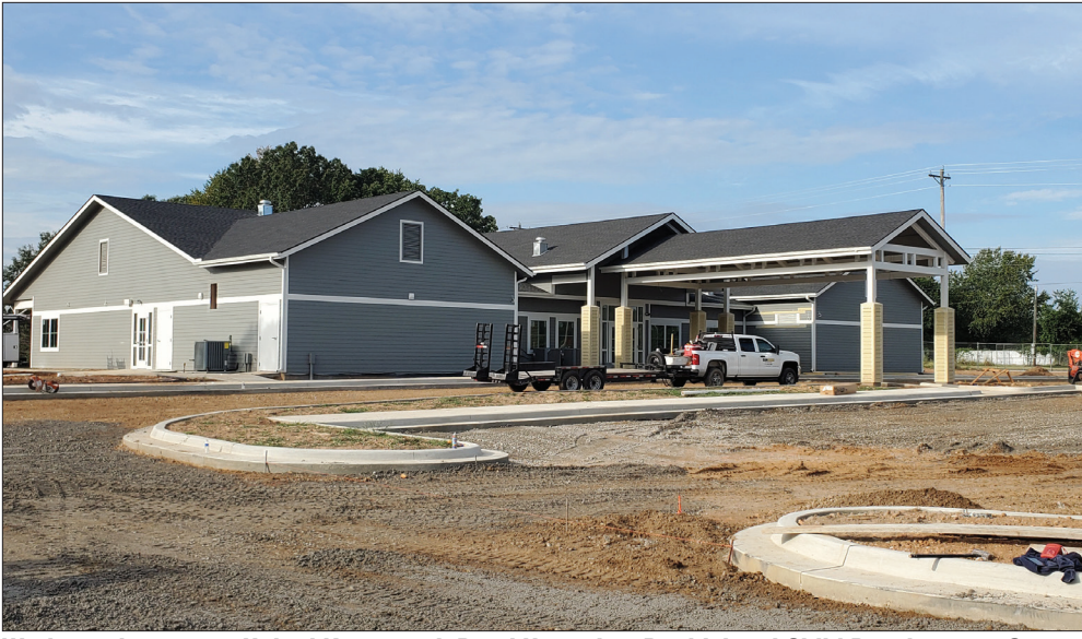
Work continues on a United Keetoowah Band Henry Lee Doublehead Child Development Center. The center opened its new expansion in August with three classrooms and a storm shelter. PHOTOS BY SHAYLEY FOURKILLER/GIDUWA CHEROKEE NEWS
