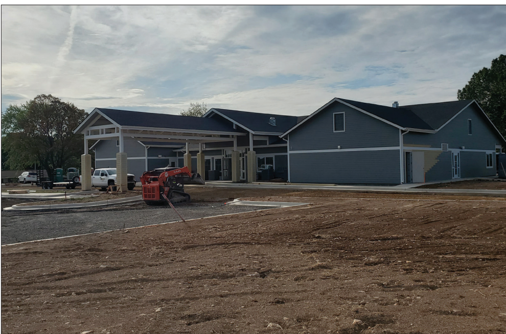
The expansion will also house three more infant and toddler classrooms. A new gross motor room, which includes the storm shelter.
